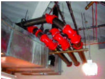
Figure 1 — The heavy pipe and short radius elbows shown in this photo had to be removed and replaced with the correct material for a beverage chase, at considerable cost.
